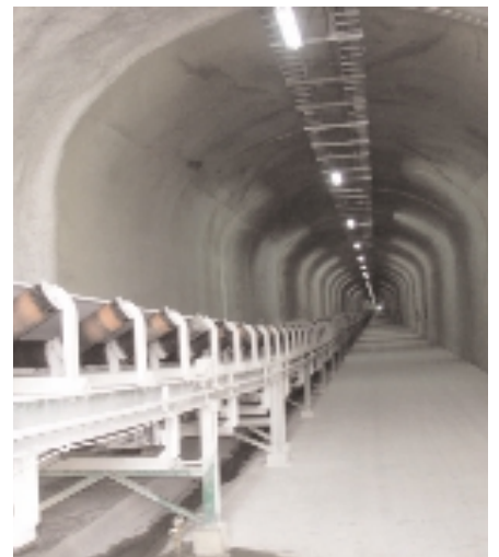
Hauling made easy: After crushing, the limestone is transported via the conveyor tunnels to a storage facility at the bottom of the hill.
