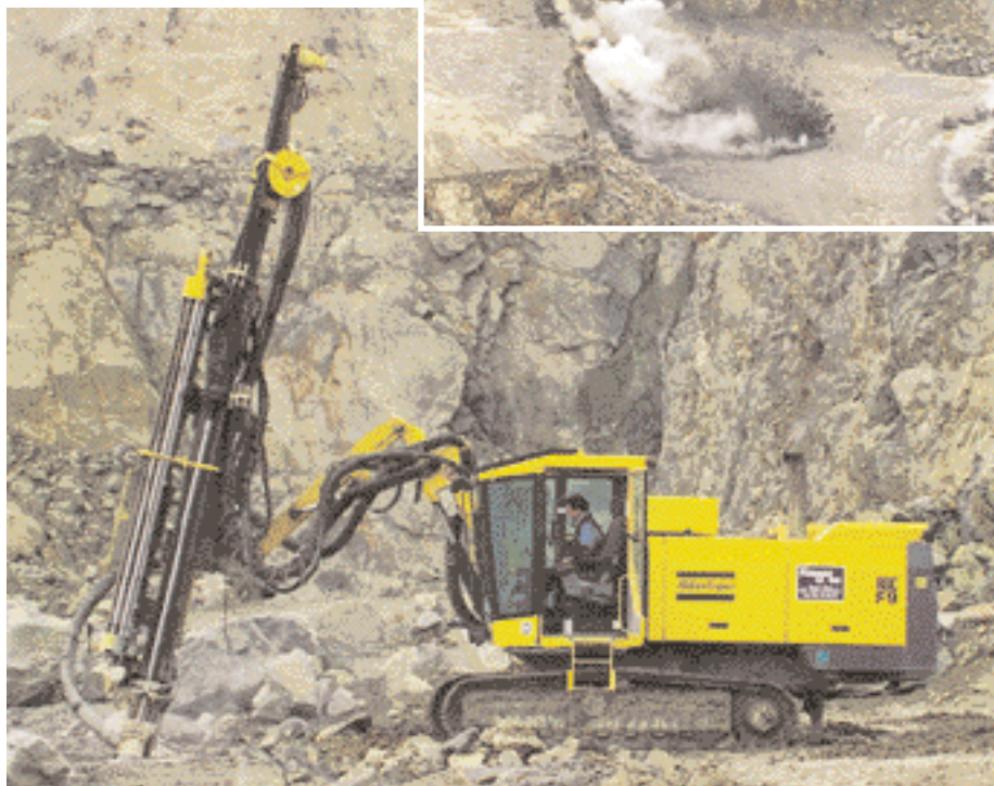
Power all the way: The new high performance ROC F9 rig equipped with the COP 2550 rock drill. The other picture (top right) shows blasting operations in one of the quarries.
