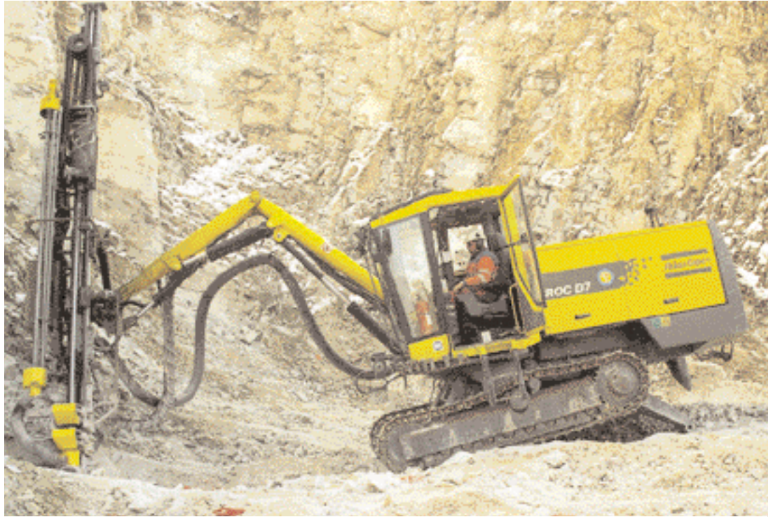
Top performance in a tough environment: The Austertana quartzite, which is hard enough to cut glass, places extreme demands on this Atlas Copco ROC D7 armed with its Secoroc drill bits.
