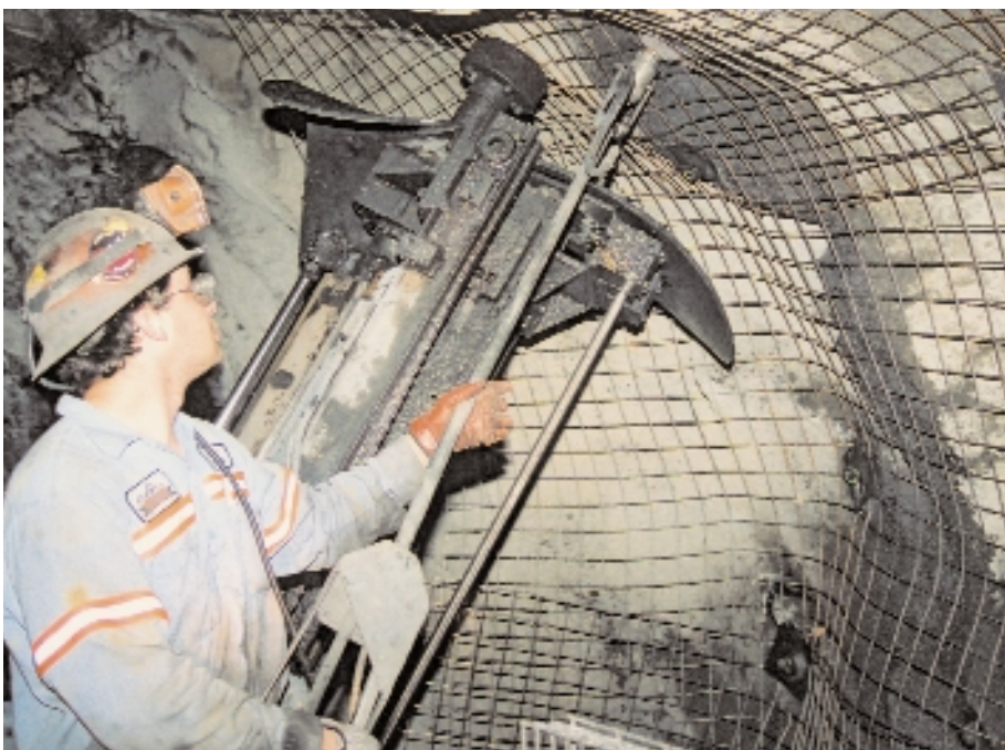
Vital operation: In the fissured and fractured rock, mesh and bolts are placed simultaneously.
