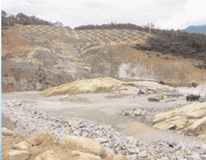
The site for the combined Hàm Thuân and Da Mi power plant on the La Nga river.
